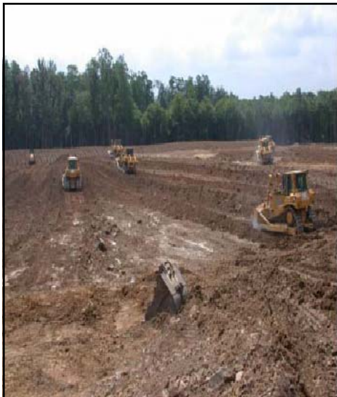
Preparation of a portion of a drilling site in Tioga County. Photo provided by DCNR.
