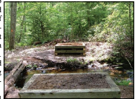
Supports for one of the new CKT bridges, constructed by the Trail Crew. Photo by Mike Kerick
